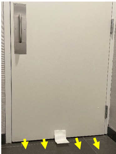
Figure 3. View from inside a negative pressure room.
