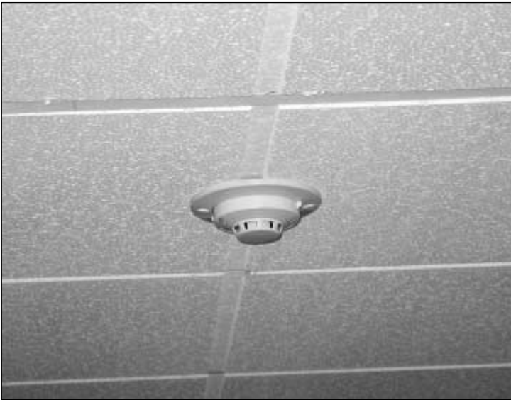
FIGURE 16.16 Smoke detector located on suspended ceiling.
