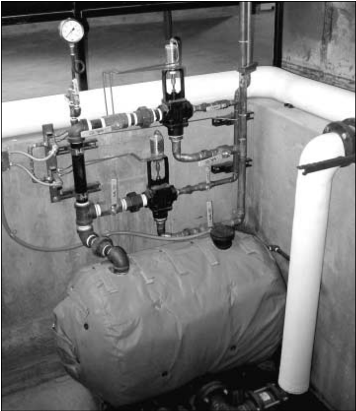
FIGURE 12.12 Condensate receiver tank, air-pump driven.
