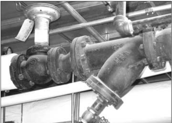
FIGURE 12.4 Steam valve and strainer.
