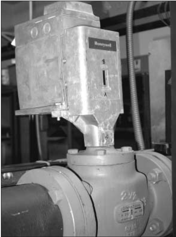
FIGURE 5.42 Electronic valve actuator and valve housing.
