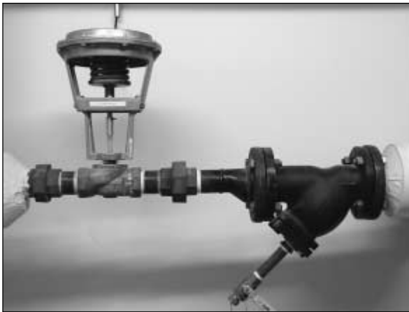
FIGURE 7.19 Strainer upstream of hot water valve.
