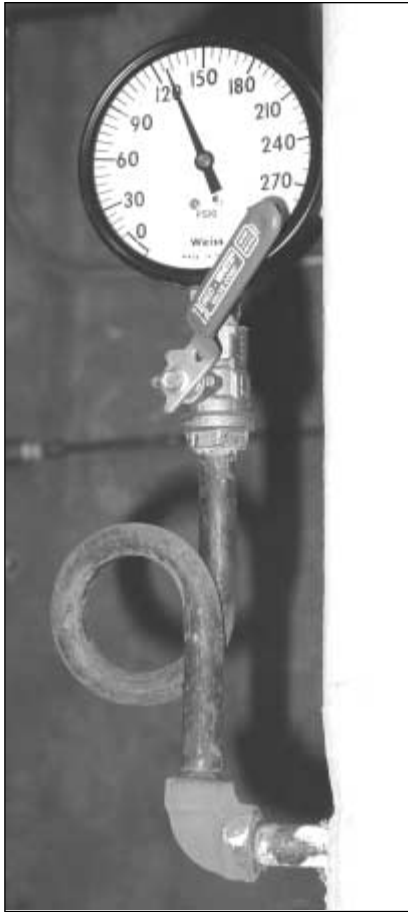
FIGURE 12.16 Steam pressure gauge with protective loop.
