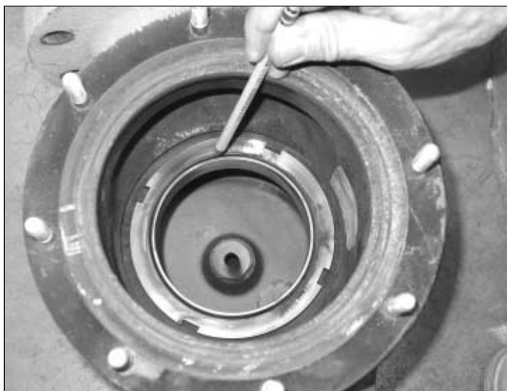
FIGURE 12.21 Valve seat on six inch steam valve.
