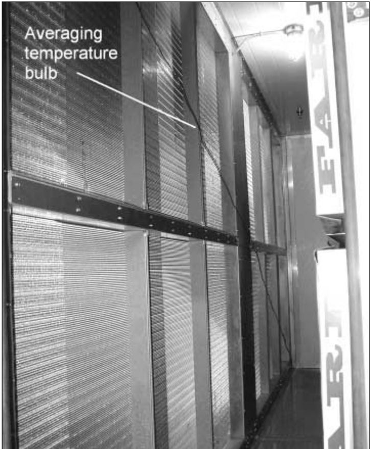
FIGURE 14.17 Mixed air temperature sensor.
