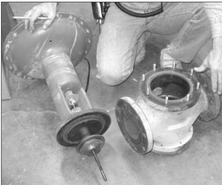
FIGURE 12.20 Six inch steam valve disassembled for rebuild.
