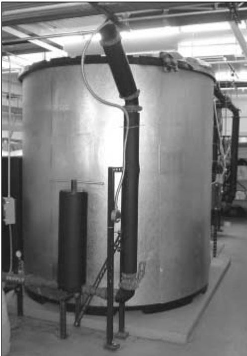
FIGURE 10.6 150 ton-hour ice thermal storage tank.
