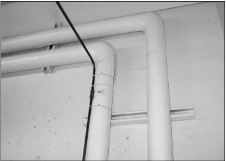
FIGURE 3.2 Insulated pipe mounted on wall brackets.
