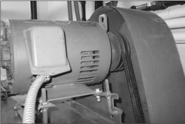
FIGURE 13.17 View of double pulley safely encased in sheet metal cowling.
