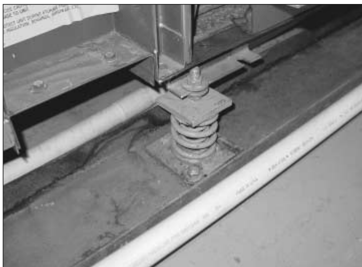
FIGURE 14.6 AHU vibration mounting.
